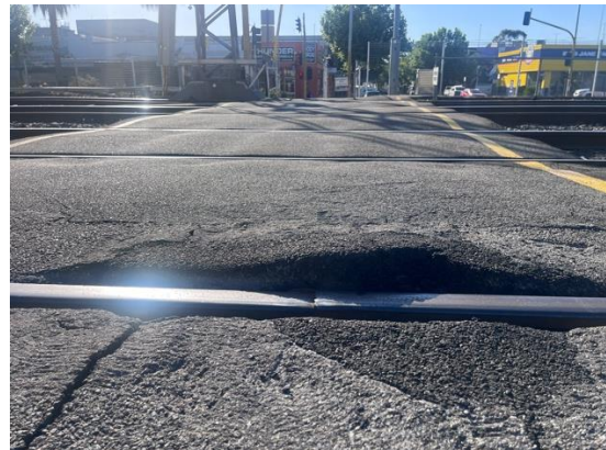
Poor levels of maintenance – trip hazards
