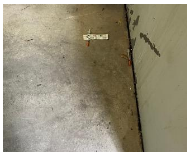
Figure 44: Syringes at base of stairwell
